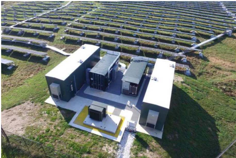
GMP's Stafford Hill Solar Farm and 4 MWh battery installation
