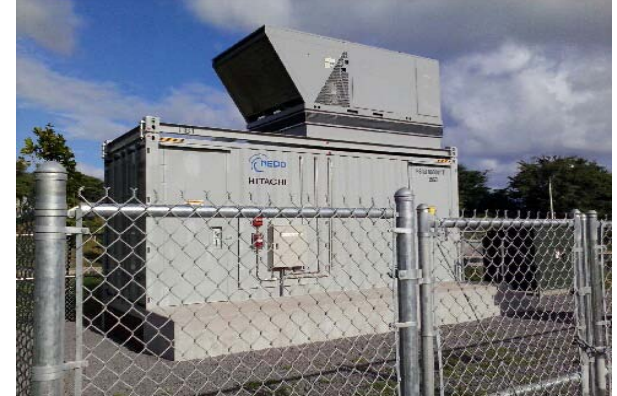
CH-75-6 120 units (153kWh)
