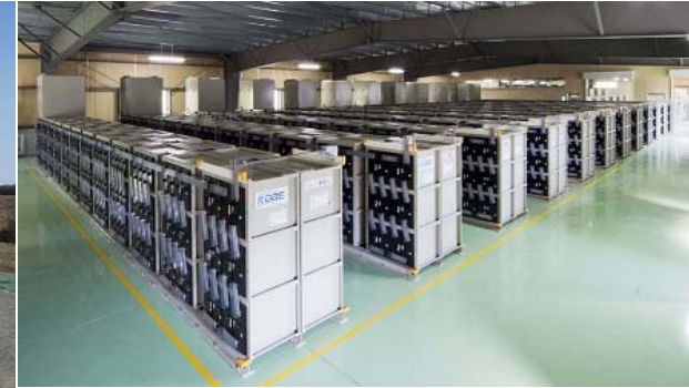
LL1500-W-8 864 units (10MWh)
