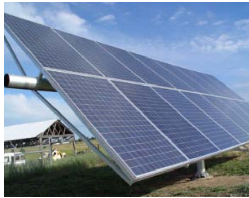
On-site generation and storage
